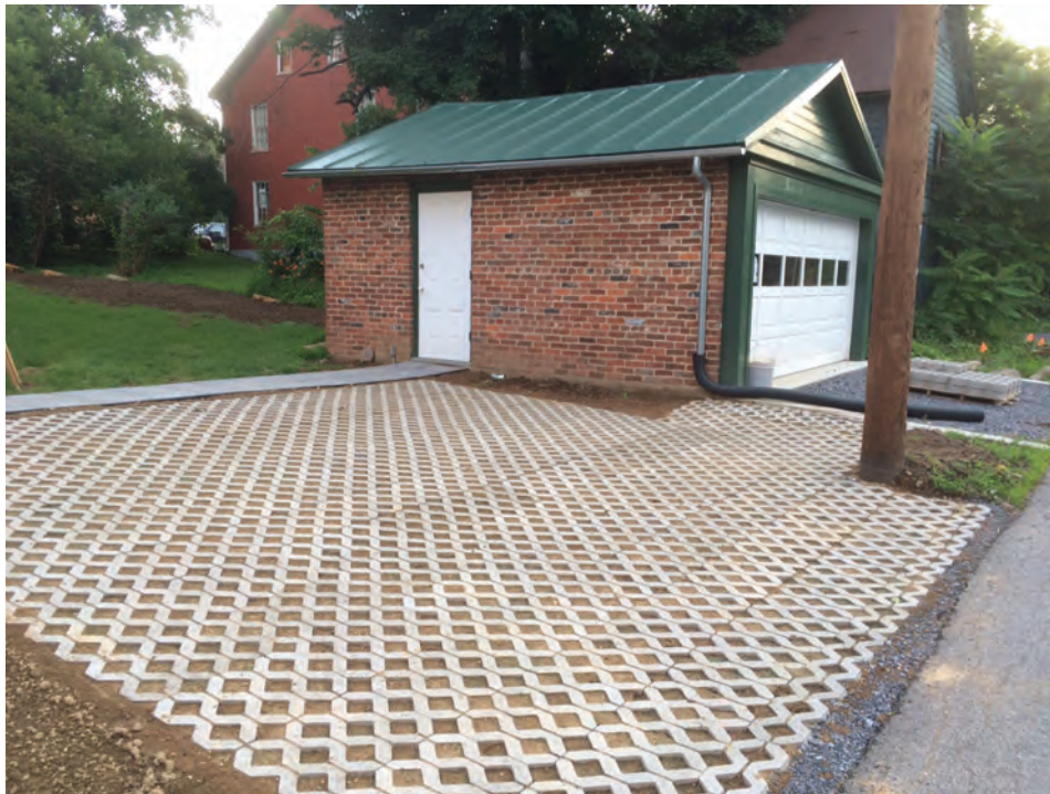
Figure 3.2. Permeable paver installation for off-street parking, prior to applying grass seed. In this situation, the downspout could be directed to the pavers since the roof is small and the runoff should be relatively clean.
